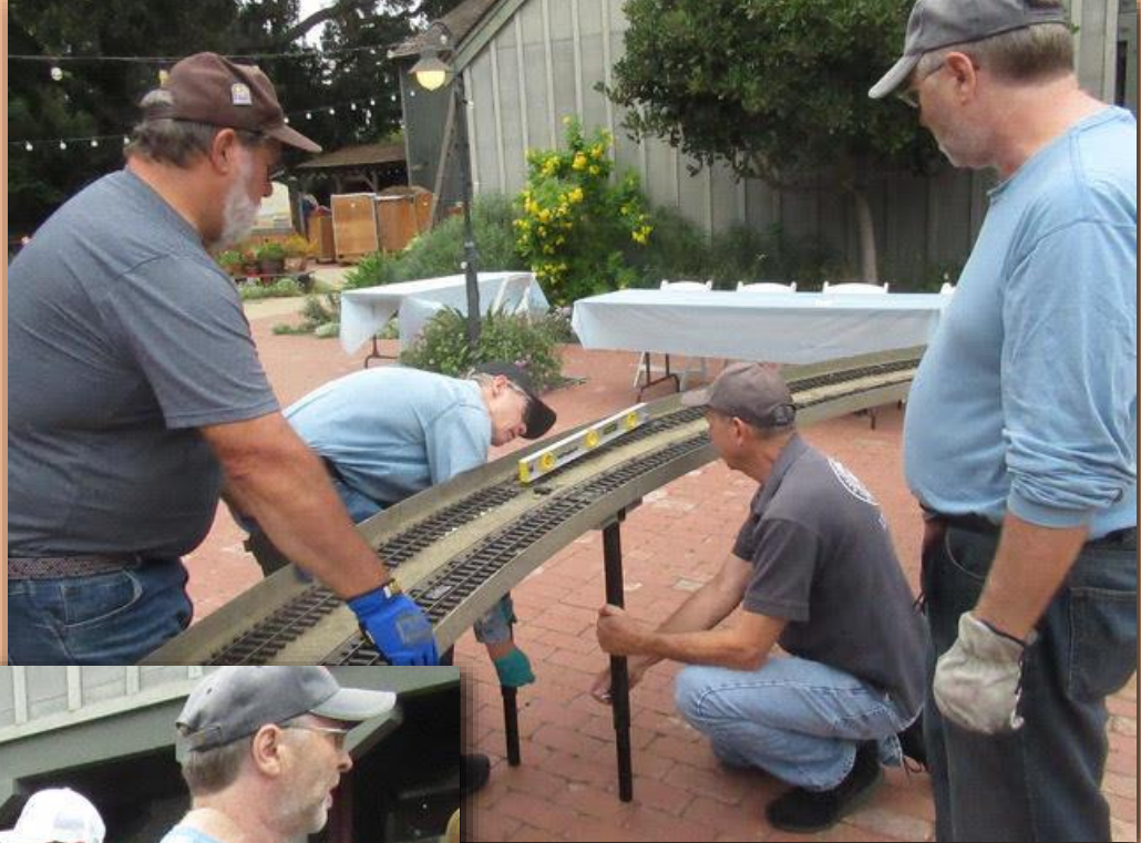
The gang levels the track. It takes almost as much time to level the track as it does to assemble it.
