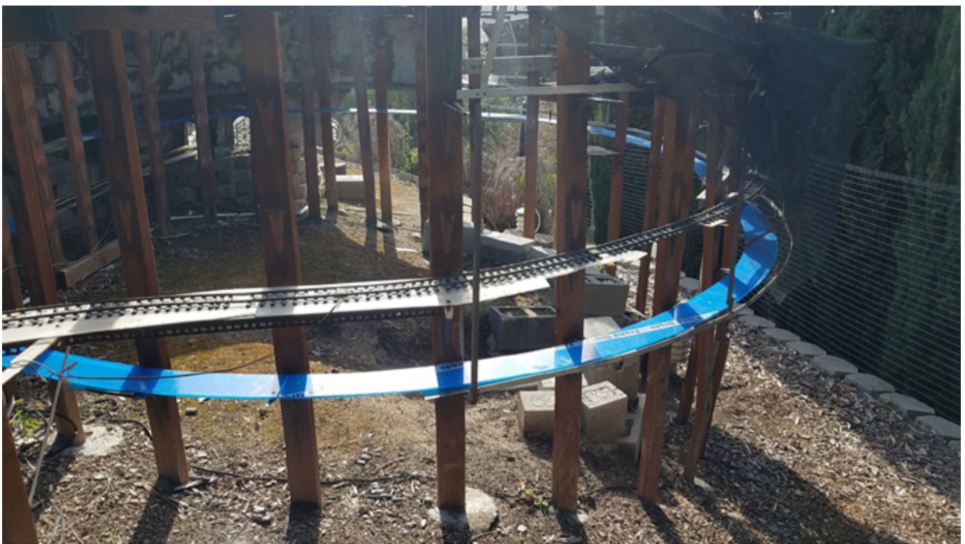
New roadbed (blue) in place provides a sturdy base for new track. Track above is only a few years old and is the return loop for continuous running.
